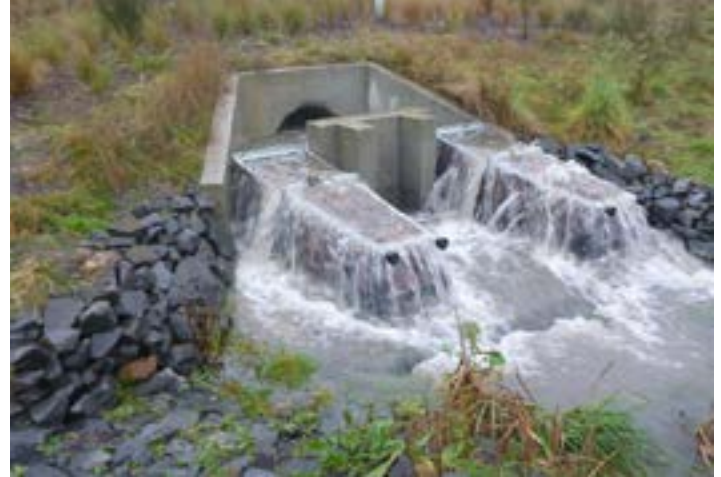
DLT 400 DUAL-WITH-DIFFUSER FULL OF GROSS POLLUTANTS
